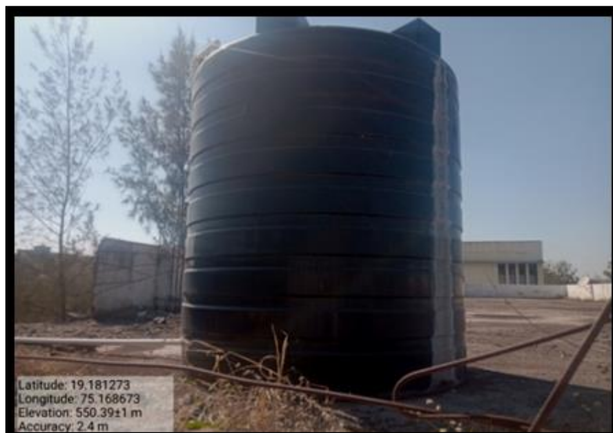
Water storage tank and water distribution pipe system
