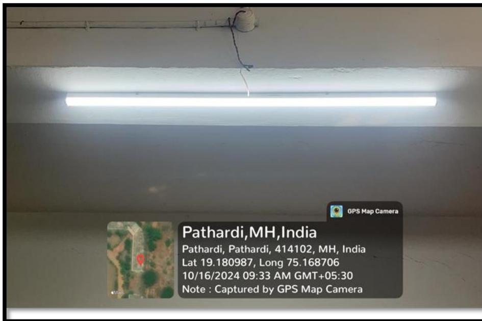
Power saving LED bulb and tubes at college
