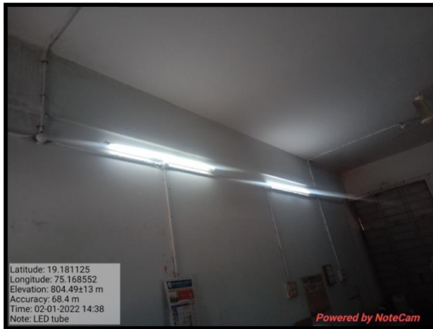
Power saving LED bulb and tubes at college
