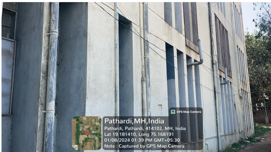
Rain Water Harvesting system at College Campus
