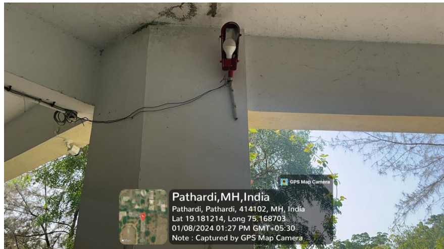
Power saving LED bulb and tubes at college
