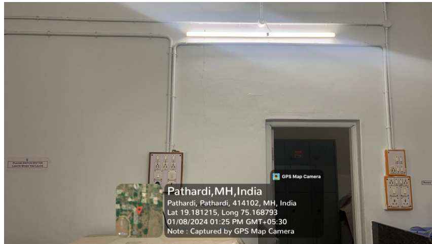
Power saving LED bulb and tubes at college
